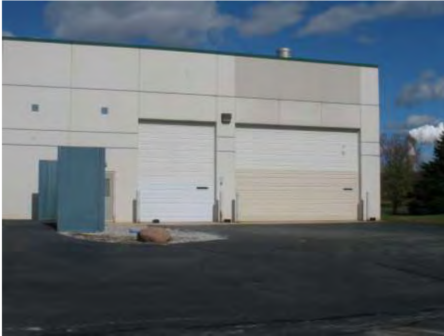
Eastern face of South Elevation; camera looking North (Loading dock area and dumpster screen)
